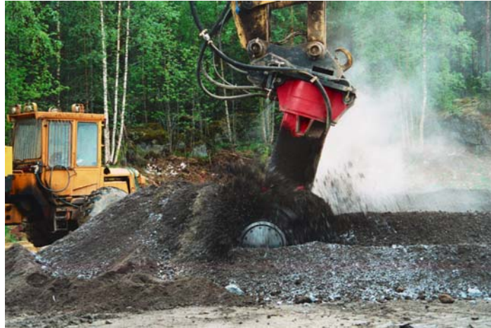
Picture 6. Mixing mass with ALLU PM Power Mix in a sport field in Luopioinen, Finland.
